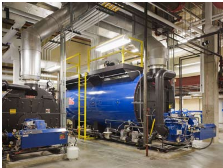
Dynamic testing of heating systems include shutting down a boiler to verify that back-up systems and alarms are fully functional.
